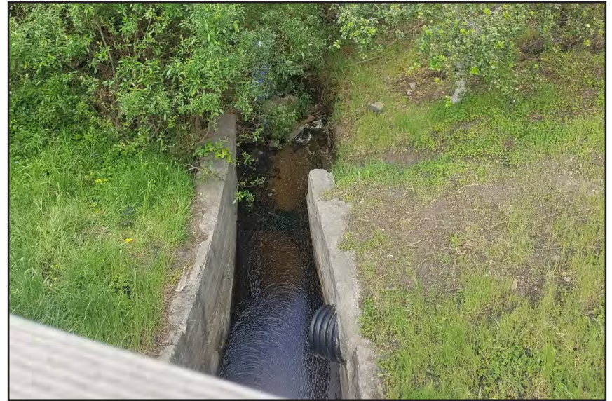
Figure 4. Standing on Pacific Street facing East, looking down at Hartnell Gulch
